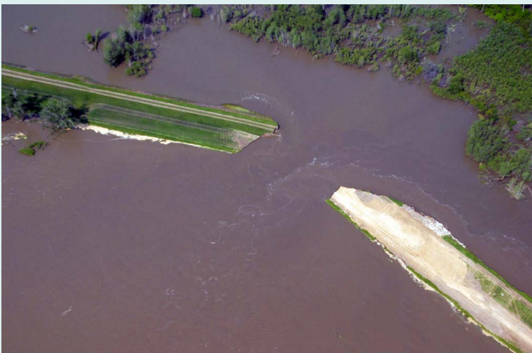
Failed levee outside Hamburg, Iowa, U.S. (Photo by U.S. Army Corps of Engineers)
